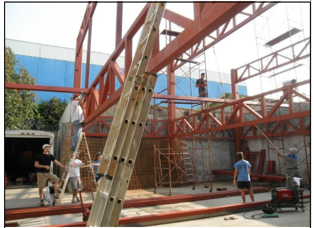
Costa Rica Steel Beams: Hoisting one of the steel beams in place for the second floor of the addition to the Iglesia Metodista El Mesias church in Alajuela, Costa Rica. (Owen Yancy, Ben McDonald, Emily Peterson, Alexa Muri, and Max)
